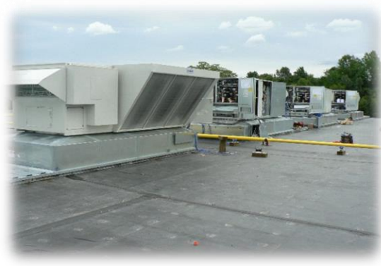
South High New Rooftop Units (2007)
