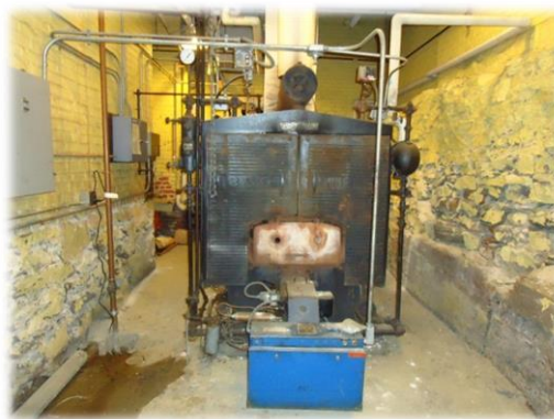
Union Hill Boiler before replacement
