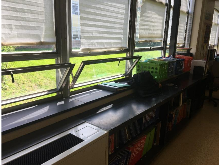
Photograph 3: Windowsill in Room 211
